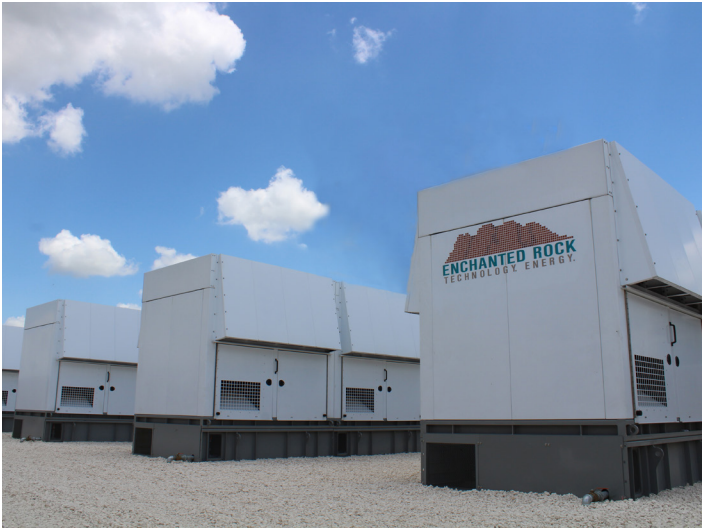
Texas A&M RELLIS Campus 10 MW
