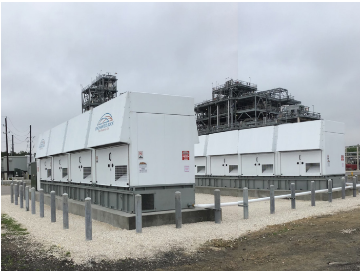
Raven Chemical Plant 3.6 MW
