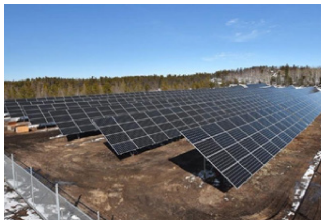
Solar panels installed in the first phase of the Three Nations Energy solar project. Photo credit: Donald Voyageur, Journal of Commerce
