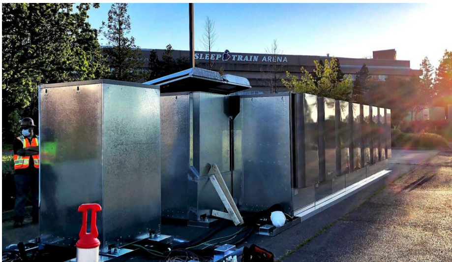
Rapid deployment microgrid being installed at the Sleep Training Arena. Courtesy of Bloom Energy
